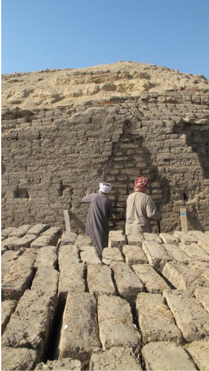
Fig. 3 Façade of the “South Palace” during filling of losses caused by looters.
